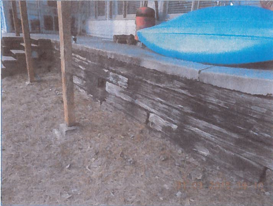
The footings, patio and retaining wall are in poor condition and are a safety issue
