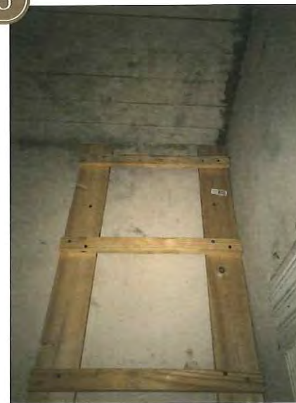
ATTIC ACCESS ALTERED TO MAKE ROOM FOR WATER EATER
