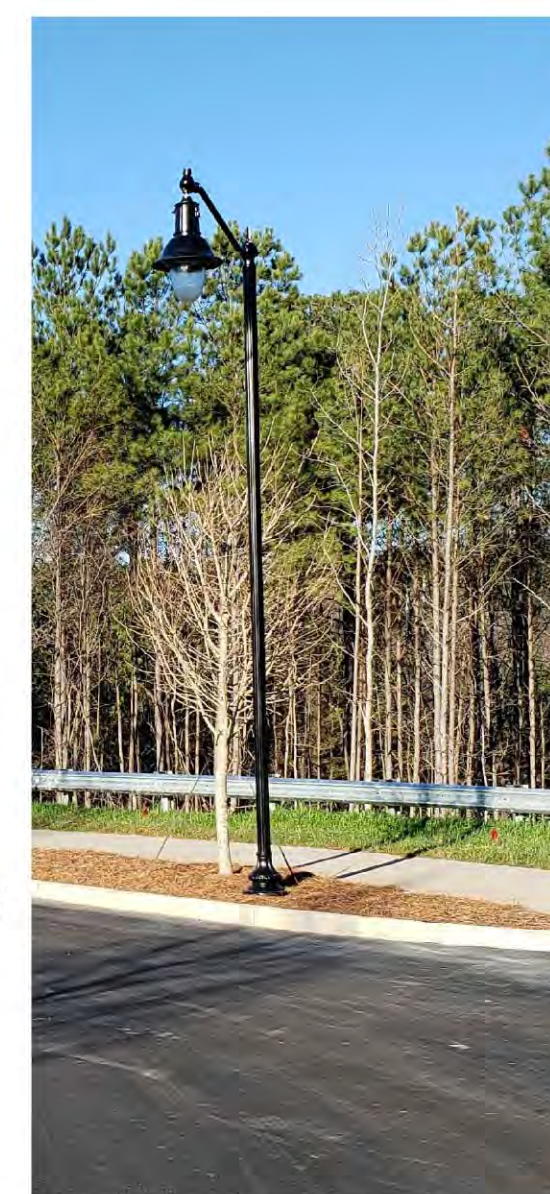
STREET LIGHT FIXTURE 20' MOUNTING HT.
