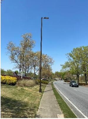
Example of existing lighting
