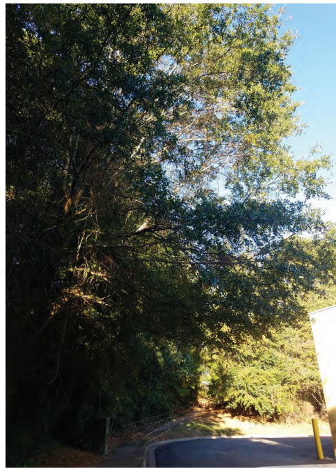
Pic # 5: Lean targeting a structure with 100% of weight over lean. Poor #5
