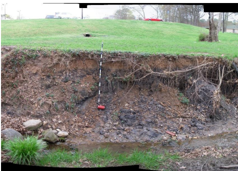
Eroded banks along reach of proposed Measure 13a
