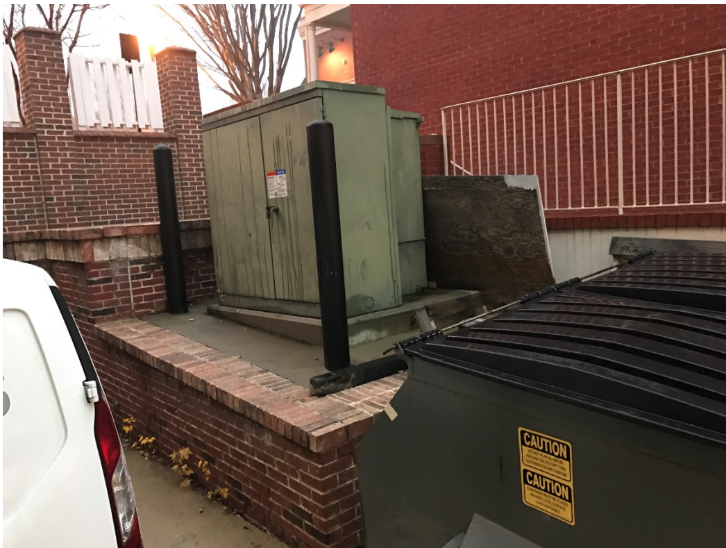
6. Existing Pad Mounted | Raised Transformer
