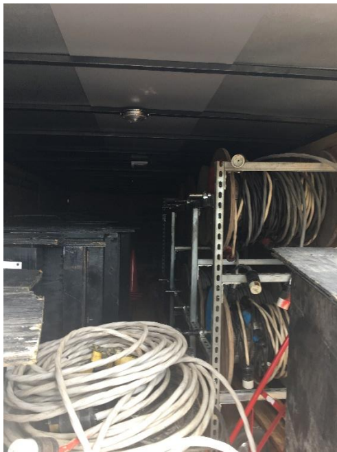
Cabling with Connectors
